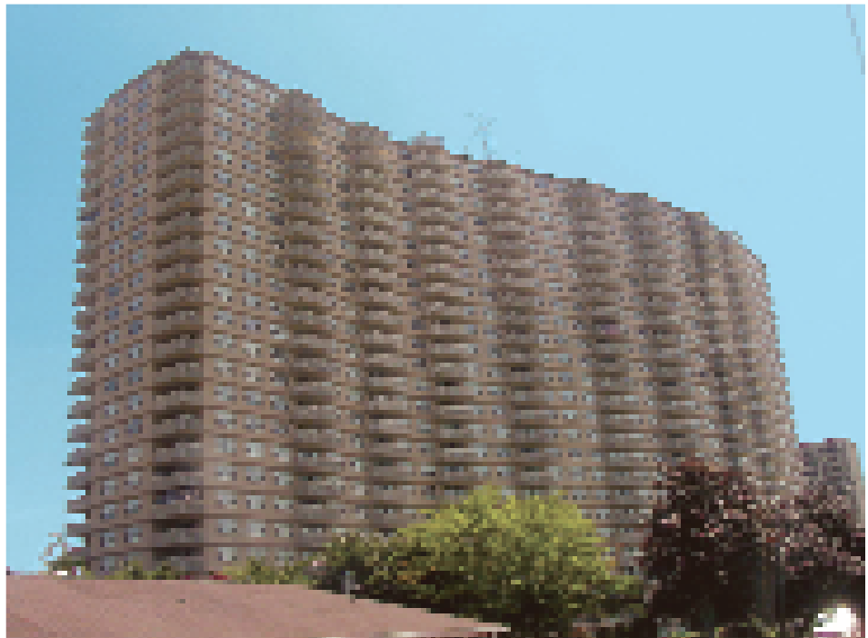
The Mediterranean Towers West, a luxury high-rise co-op apartment building in Fort Lee, New Jersey, upgraded its fire alarm system with a Silent Knight IFP-1000 integrated voice evacuation system and addressable fire control panel, and new alarms in every unit.
