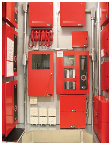
Part of the extensive product installation at the Plaza.
